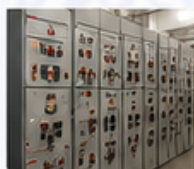
Control & Distribution Panels
