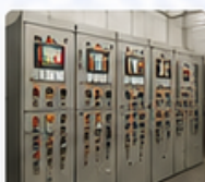
Control & Distribution Panels
