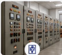
CONTROL & DISTRIBUTION PANELS
