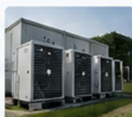
HVAC & Building Management Systems
